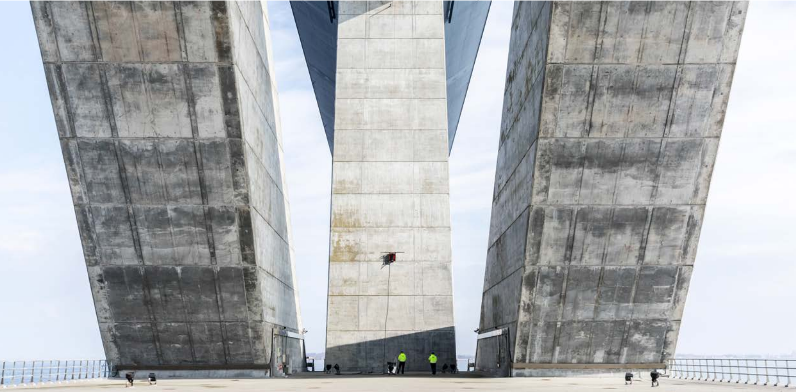
FORCE Technology works closely with the Danish offshore industry in several areas including inspection of bridges, wind turbine blades and other hard-to-reach locations.
